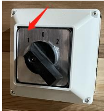
Power to stove heater
