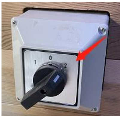
Power to Infrared heaters
