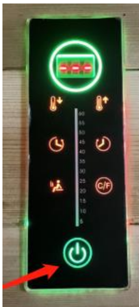
Sauna Control Panel is Illuminated
