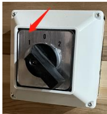
Power to stove heater
