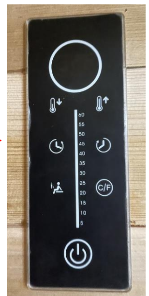
Sauna Control Panel has no Illumination
