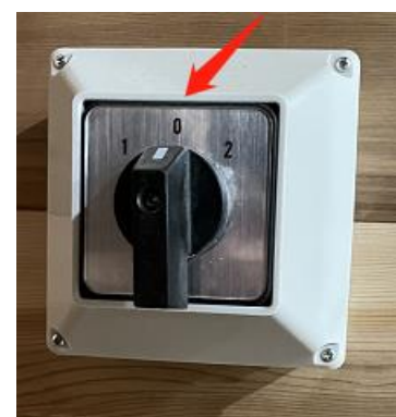
Power turned OFF
